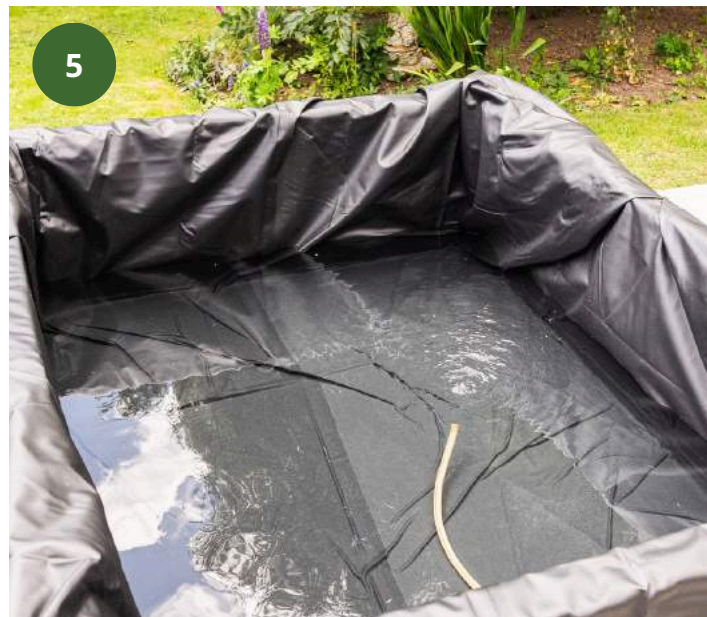
Start filling with water - let the liner find its natural position within the structure as it fills with water.
